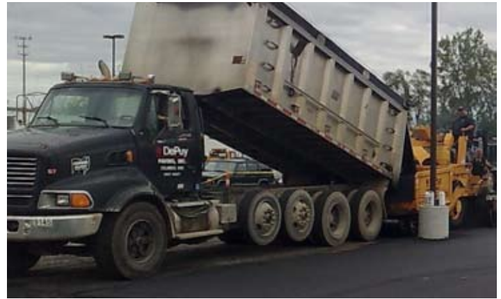
DePuy Paving, is doing the final paving repairs for this year. These paving repairs on the west and south side should be finished by Nov. 14. The repaired areas also will be restriped.
